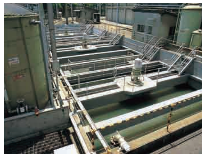
廃水中和処理槽 Tank for neutralizing waste water
